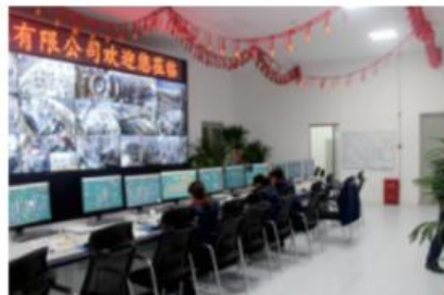
central control room
